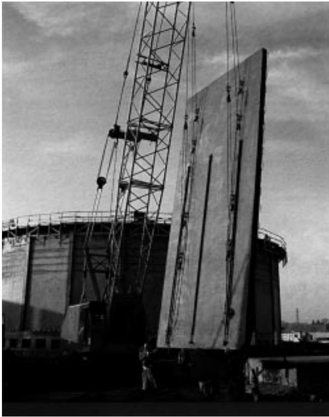
A 150-ton track-mounted crane with an eight-point lifting pick erects tilt-up concrete panel at Bissell Point WWTP.
